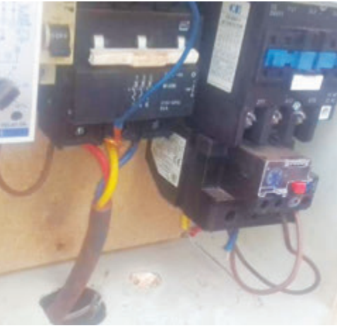
The cable to the booster pump was stolen by criminals.
